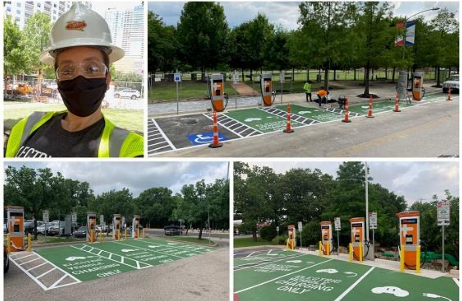
Clockwise from top left: Shems Duval project managing a site installation, Electric Drive, Mueller location and Austin High School location.
